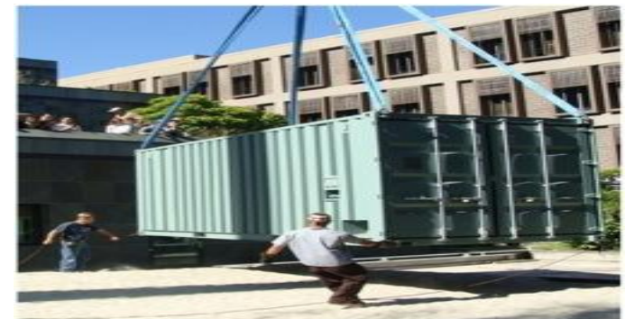
The Million Server Datacenter Providing IaaS
